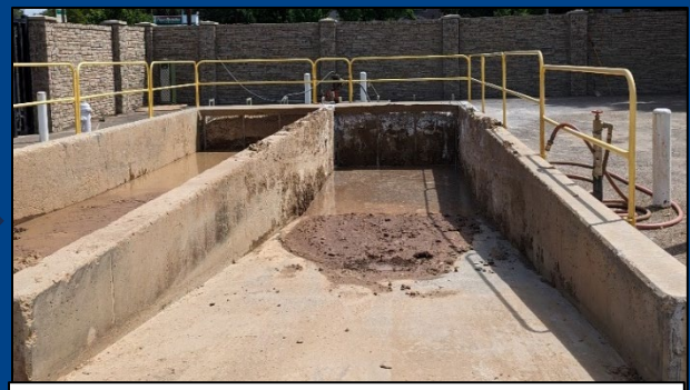
The vacuum basin can then be cleaned out and the dirt can be disposed.
